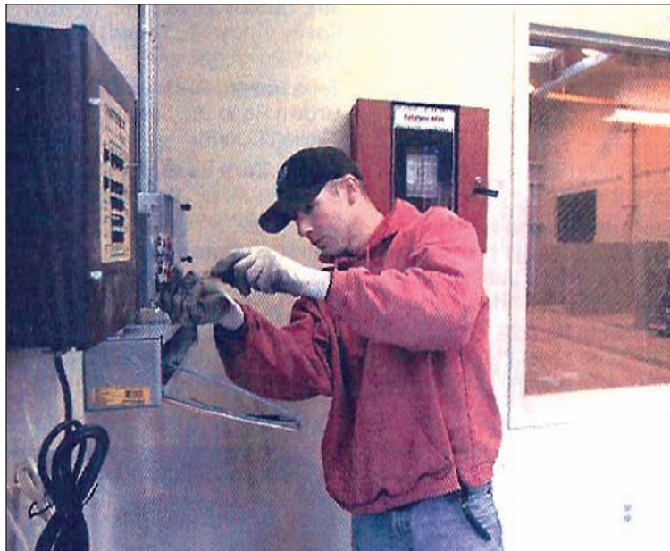
Scott Gatchet of EC Electrical Construction Co. works on wiring for the household hazardous waste facility.
